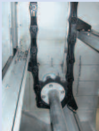
Sludge skimming system and pressurised water supply
