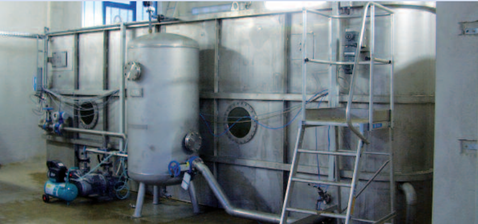
Flotation unit with pressure tank
