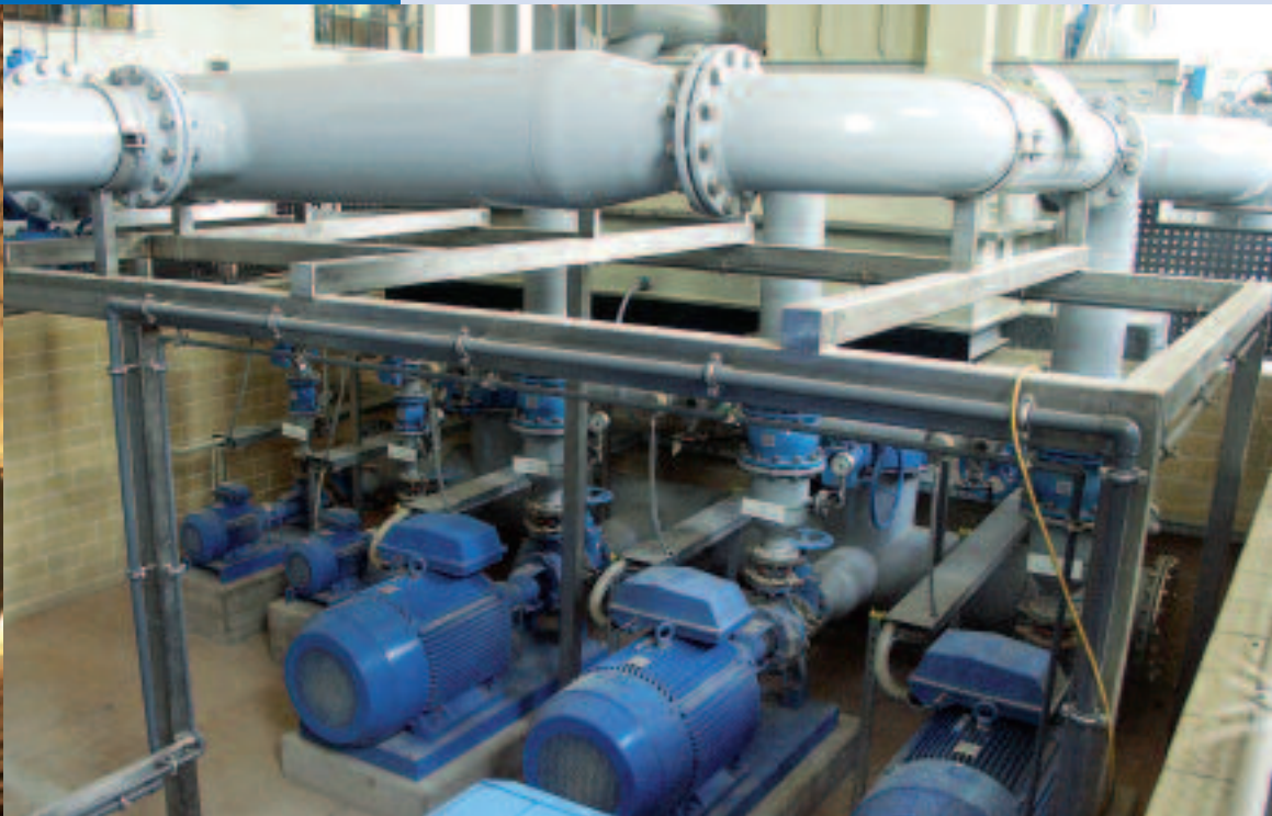
View of the trickling unit for neutralising the water.
