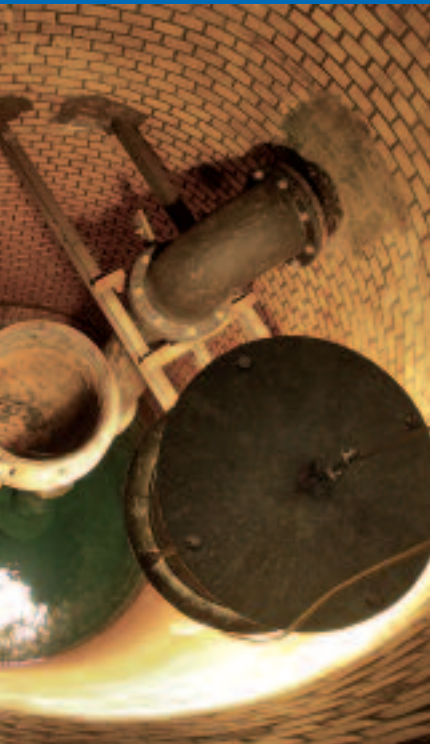
One of the seven wells with pump for raising the raw water.
