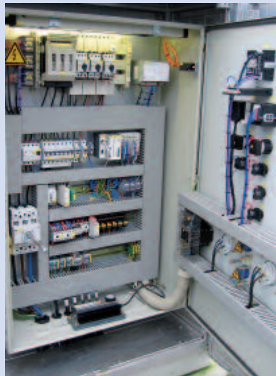
Monitoring of an outlet construction with a TeleMatic Controller type SMART-400.
