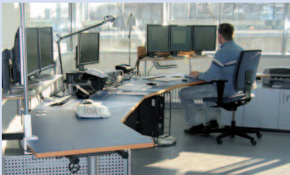
In the Greffern control centre, a two-computer process-control system was installed with redundant operating stands. The two operating stands each consist of three TFT displays for overview and individual-plant images as well as graphics and reports.
