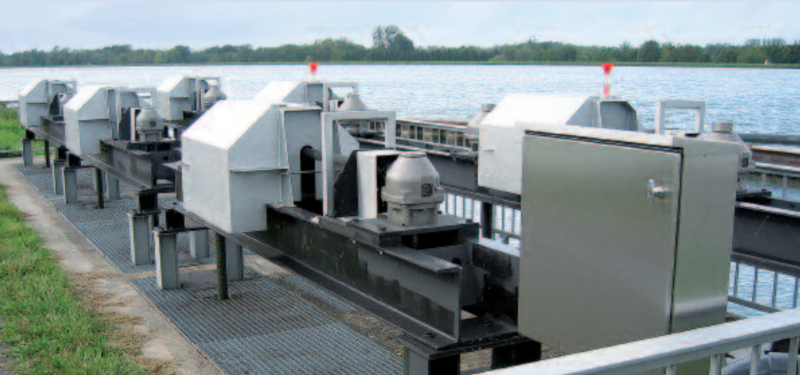
Driving machines for the three shields on the surge construction in sub-polder 2.
